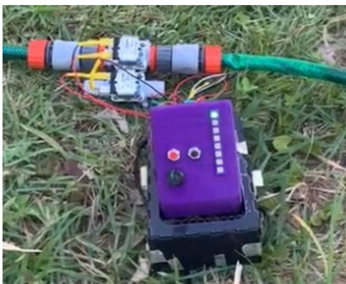
Figura 12 - Painel integrado as válvulas e as mangueiras
